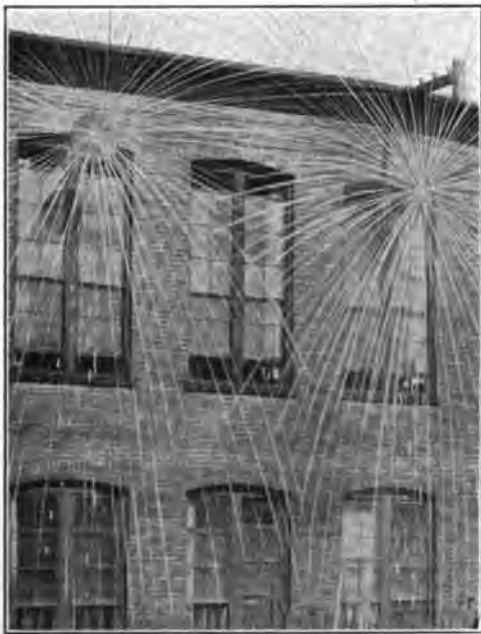
SPRAY FOR COOLING MILL.
